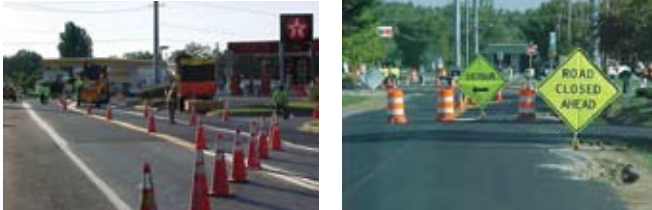
Traffic control provided by the Centreville maintenance team with only a one-day detour for drivers
